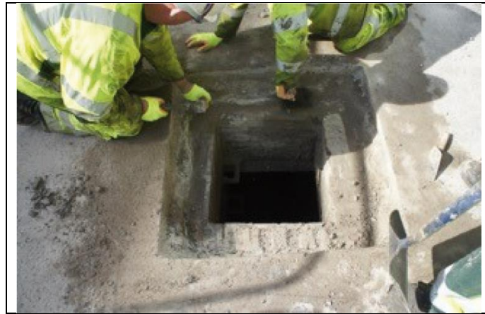
Figure 1 Preparation of damaged ironwork (from site visit)
