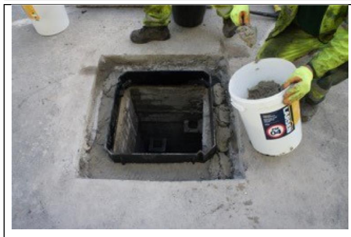
Figure 1 Preparation of damaged ironwork (from site visit)
