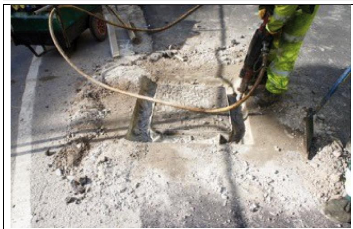
Figure 1 Preparation of damaged ironwork (from site visit)
